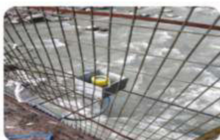
Automatic Water Level Recorder Sensor
