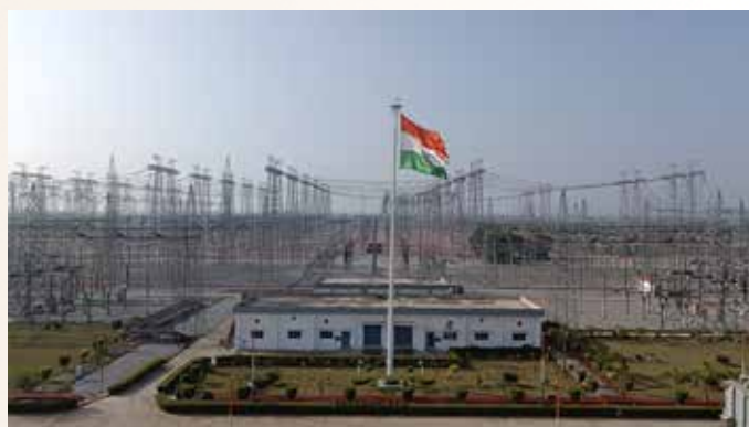
Agra HVDC Substation
