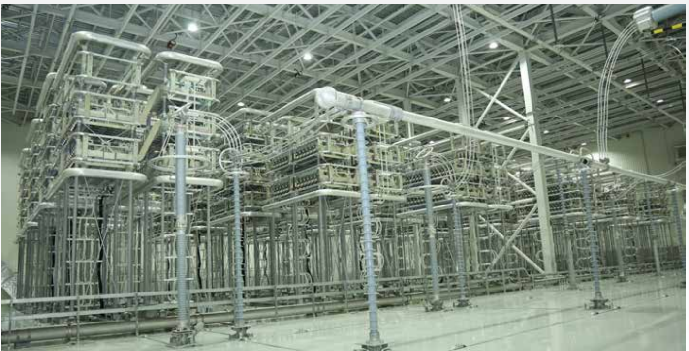
Valve Hall: Raigarh-Pugalur-Thrissur 6000 MW HVDC system
