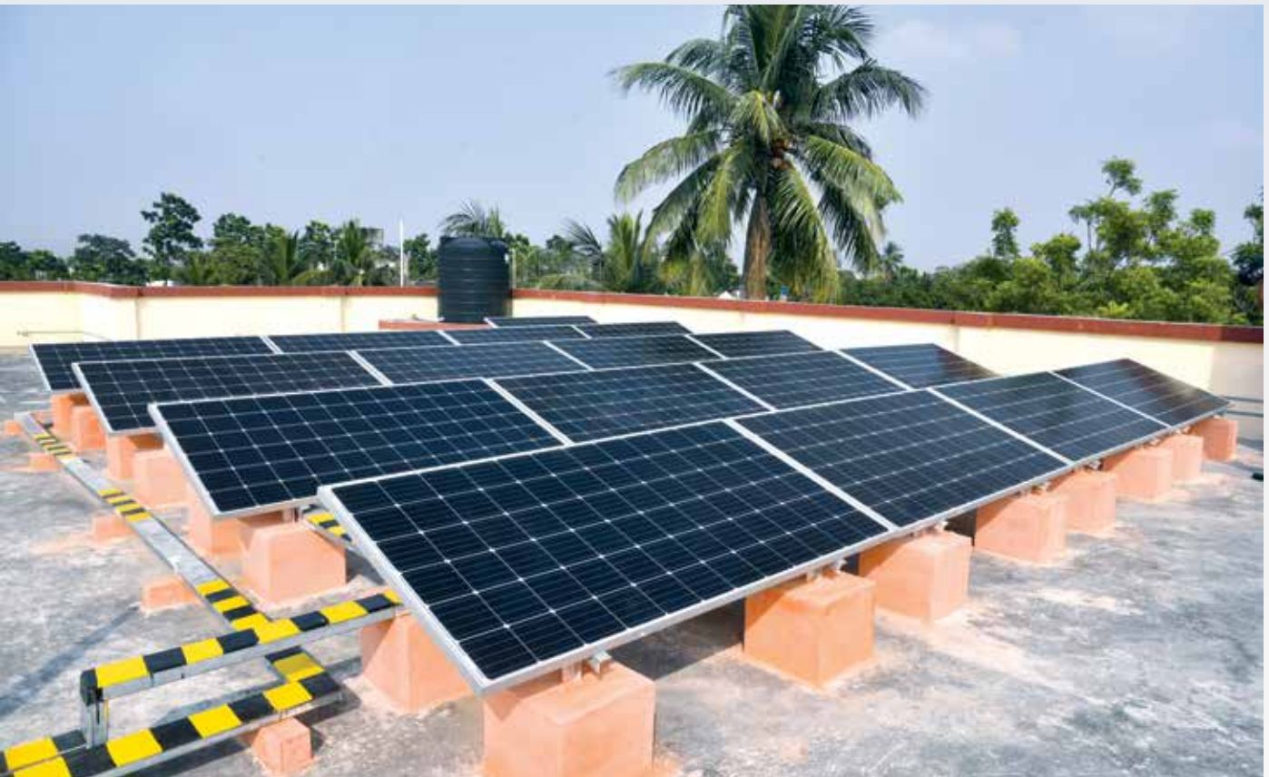
Roof Top Solar DVC
