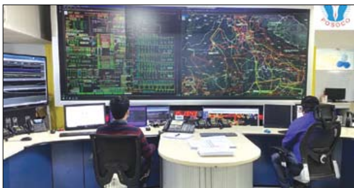
National Load Despatch Centre Control Room
