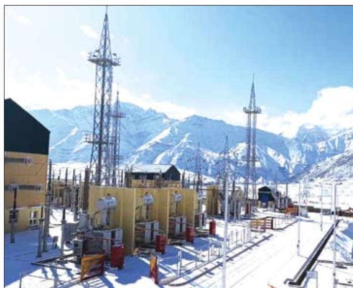
220 kV Phyang, Leh substation
