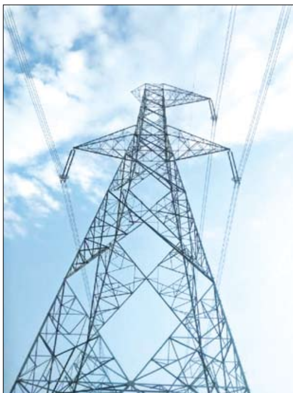
Ghatampur Transmission Line funded by PFC
