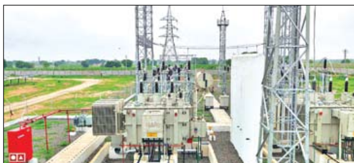
Switch Yard at 40 MW Bhordu Site funded by PFC
