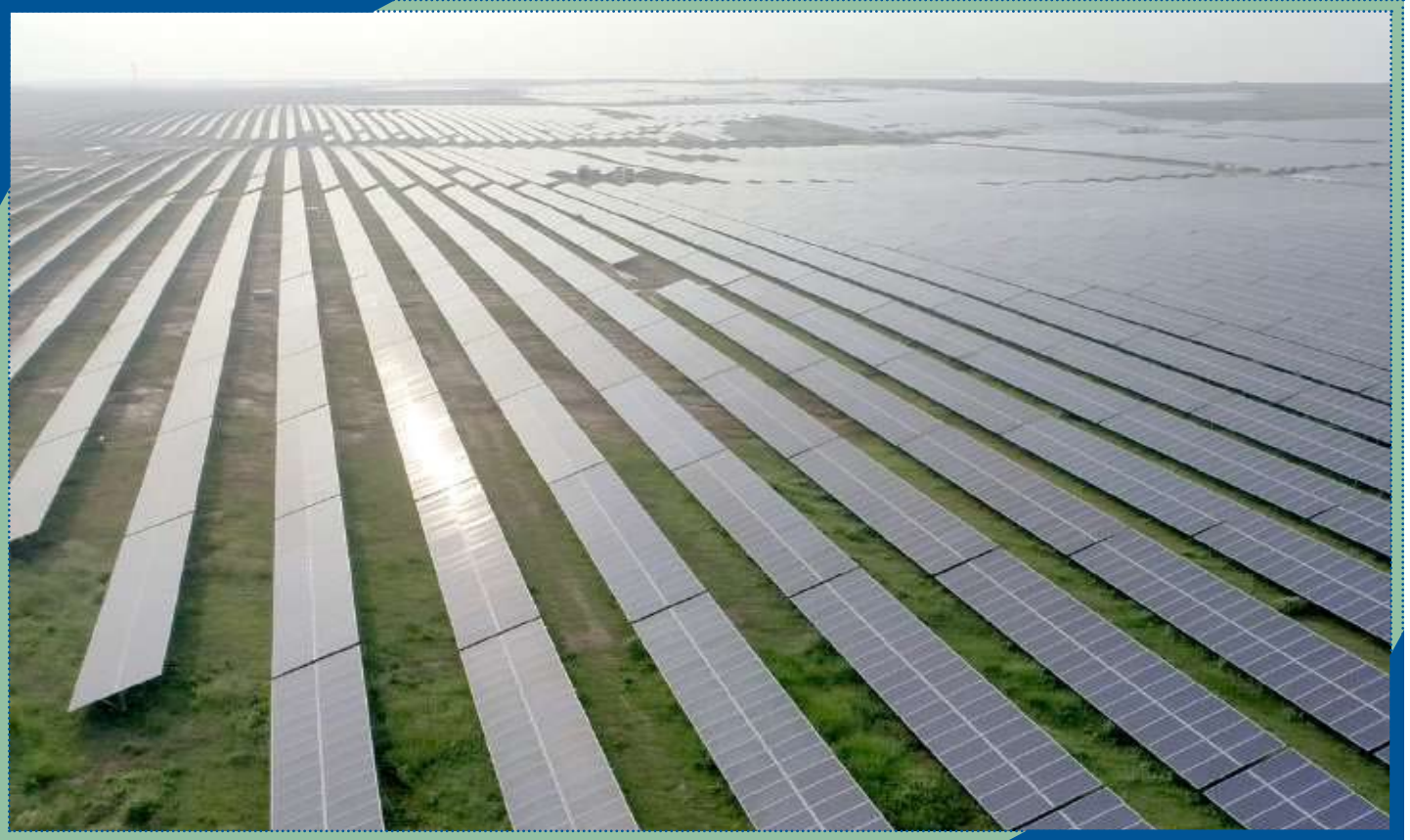
750 MW Rewa Solar Park, Madhya Pradesh
