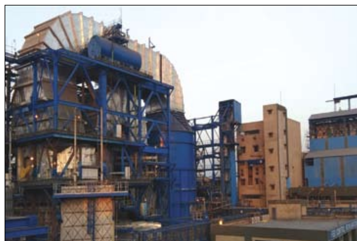
FGD system installed at NTPC Vindhyachal TPS
