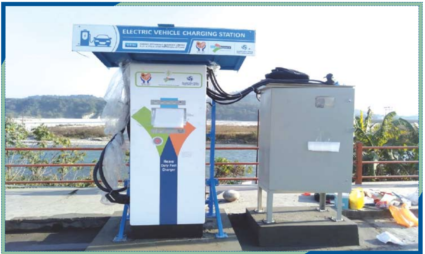
Electric Vehicle Charging Station, Haridwar (Uttarakhand) by THDCIL on 06.01.2022 for public convenience under CSR
